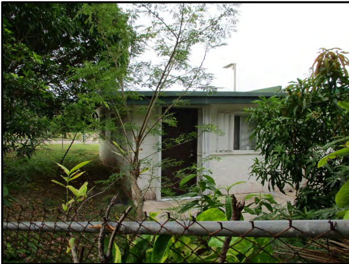
Photograph 7. The adjoining property to the south also contained two single-family dwellings (14 March 2019).
