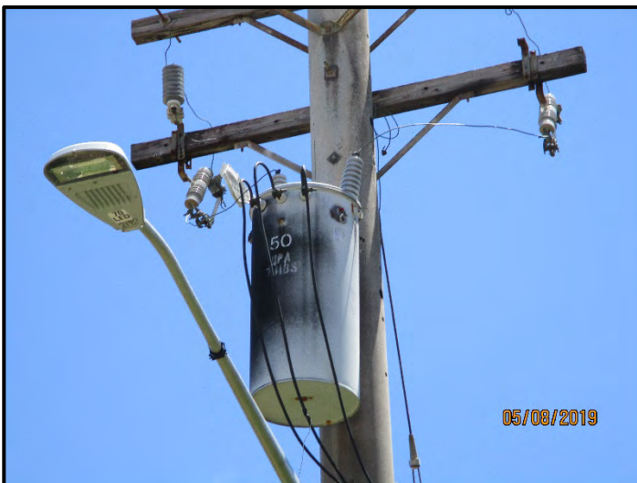
Photograph 18. One pole-mounted transformer was observed to the south of the subject property, along Atbut Lane and at an apartment building. Black staining was visible on the exterior of the transformer (09 May 2019).
