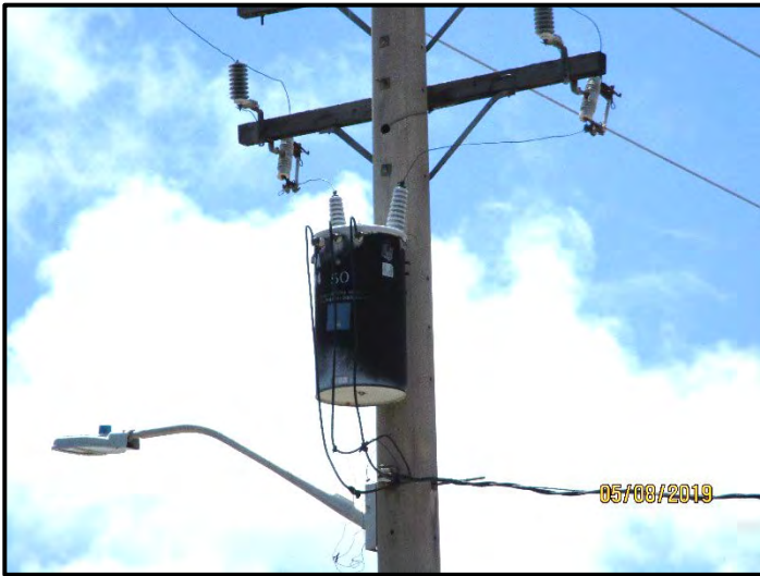
Photograph 17. One pole-mounted transformer was observed to the northeast of the subject property, along University Avenue. Black staining was visible on the exterior of the transformer (09 May 2019).
