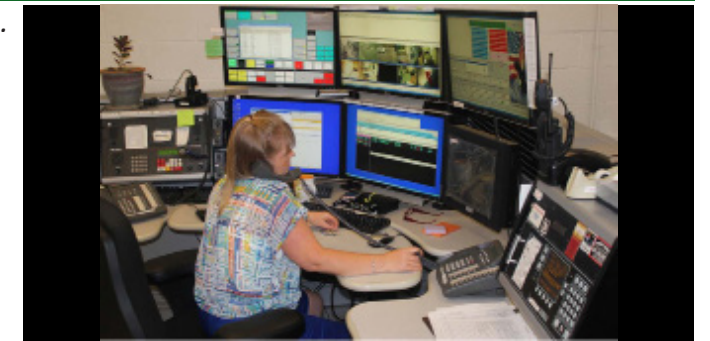
An example of an emergency communication hub.
